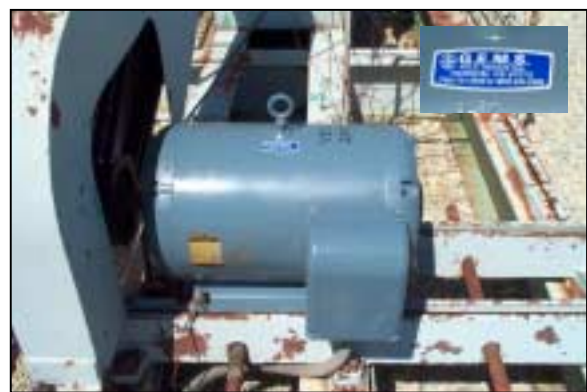
The test well Lufkin pump jack is powered by a rewound 20 hp Baldor motor. Vess Oil takes power at a substation approximately a mile from the well and manages distribution in the field.
