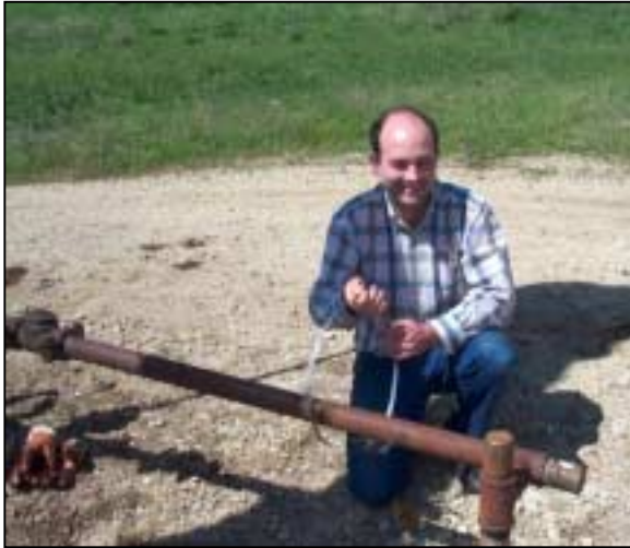
The flow pipe was clean and the flow sensor attached with a hose clamp and contact gel.
