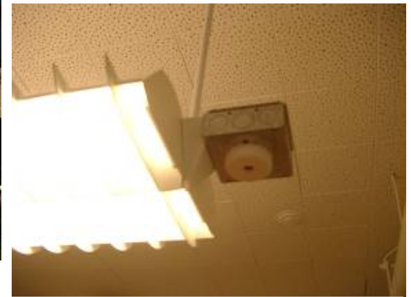
Photosensor built into luminaire
