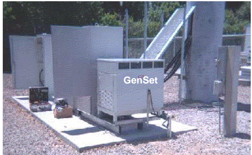
Small Remote Telecommunications
