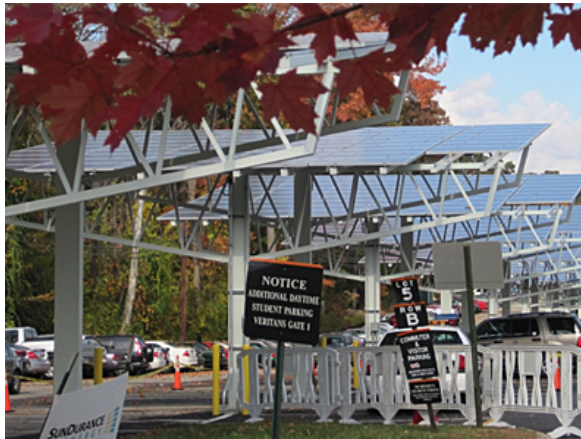
A solar farm at William Paterson University is expected to generate up to 20 percent of the school's electricity. | Photo courtesy of Energy Blog
