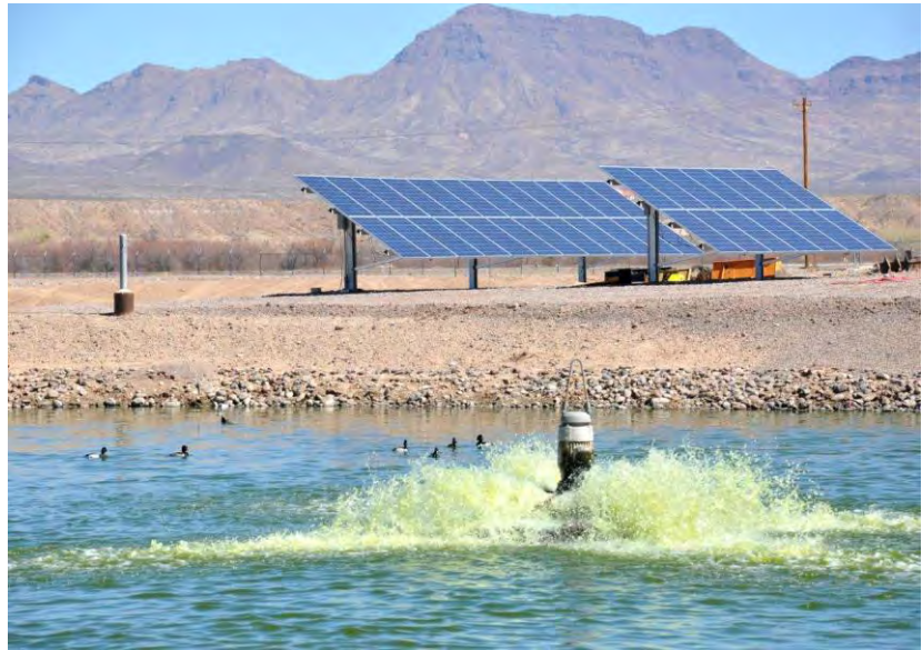
Solar powered water aerator in a wastewater facility in the Town of Thatcher, Arizona as part of SunPumps of Safford’s 21 st Century Energy Demonstration Project.
