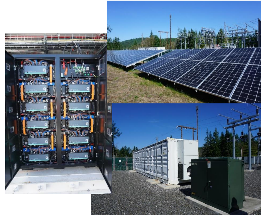
OPALCO – Solar & Energy Storage $1.0M & $2.4M
