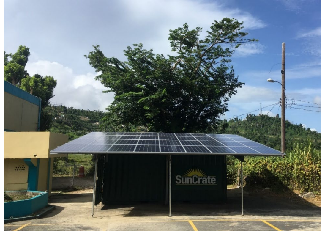
Earlier microgrid: Solar crate in Puerto Rico, August 2018
