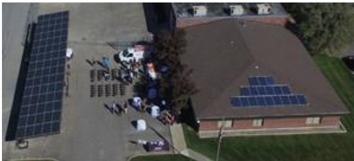
Completed in October 2015, this Utah C-PACE project installed a solar canopy, microgrid, and electric vehicle charging station in Hunt Electric's West Valley City headquarters. Photo courtesy of the Utah Governor's Office of Energy Development.
