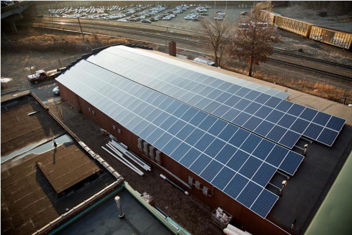
Crest Mechanical in Hartford, Connecticut used $145,000 in C-PACE financing to install a 44 kW solar photovoltaic system. The system will save over $400,000 in energy costs over the life of the equipment. Photo courtesy of the Connecticut Green Bank.
